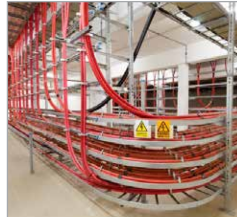
Athens International Airport, Power quality optimization system
